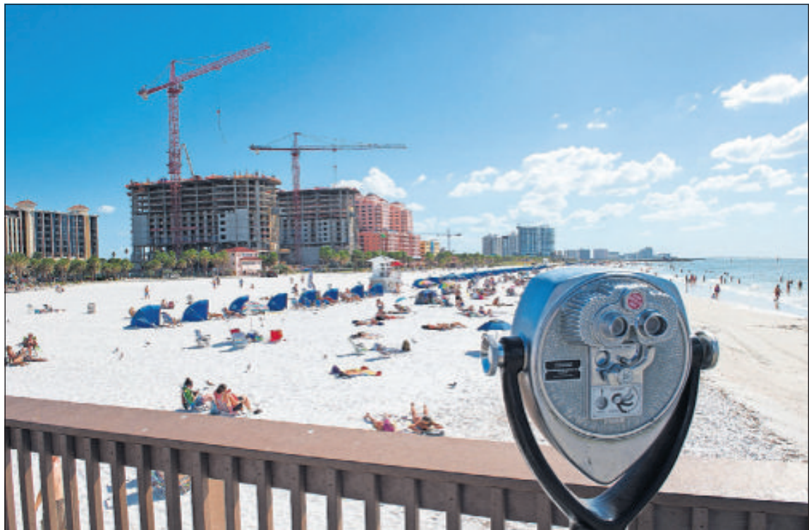
The Wyndham Grand Resort Clearwater Beach that is expected to open in early 2017, located at 100 Coronado Ave., Clearwater Beach. It overlooks Clearwater Beach. STAFF PHOTO / THOMAS BENDER
